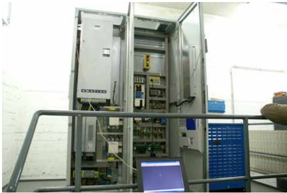
Image 6 Control system: The new control cabinet with the DC power supply and the elevator control unit.
