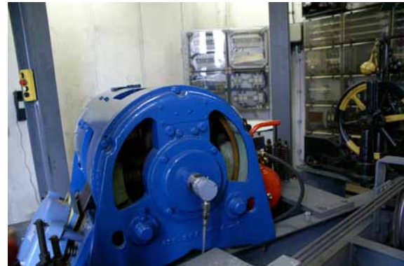
Image 7 and 8 WDG/From above - engine room: The Wachendorff Automation encoder at its operating site high over the roofs of the city.
